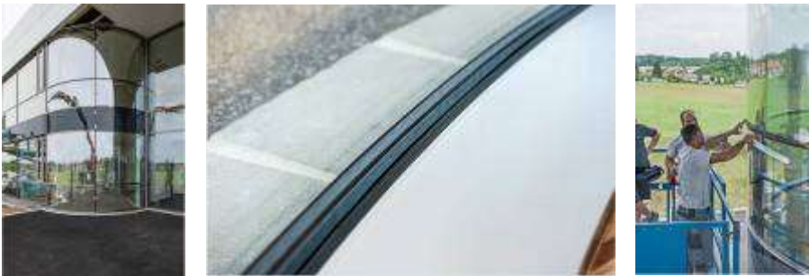
Photos 11, 12 and 13: The precisely fitted insulating glass elements are then permanently connected to the supporting sub-construction using aluminium trims.
