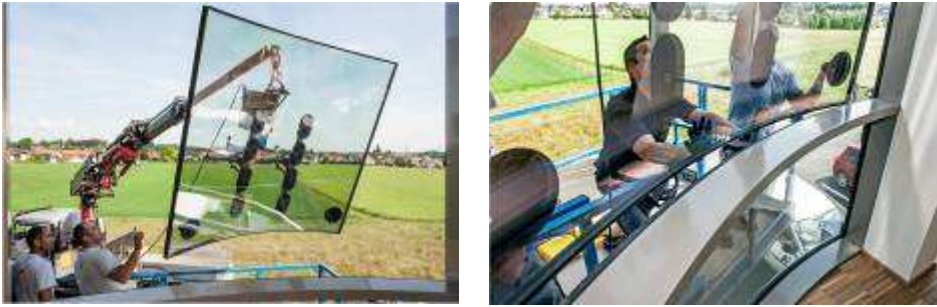
Photos 9 and 10: The curved facade elements made of triple insulating glass are lifted with the aid of a crane and placed in position from the raised platform.
